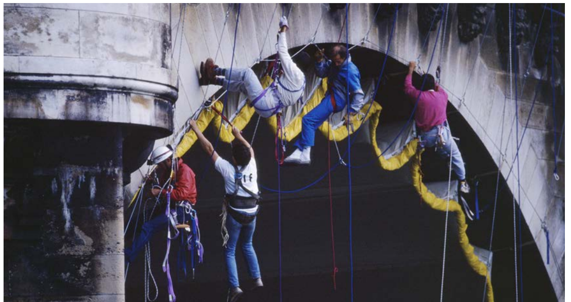
12 Climbers attach the fabric hoisted under one of the arches and adjust the tension of the straps sewn onto the fabric, making it hug the lines of the vault [September 16-22, 1985].
